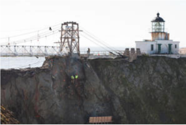
Point Bonita Lighthouse bridge undergoing construction in the Marin Headlands in Sausalito. Construction is expected to be finished by April 1, 2012. (Special to the IJ/Meghan Roberts)
