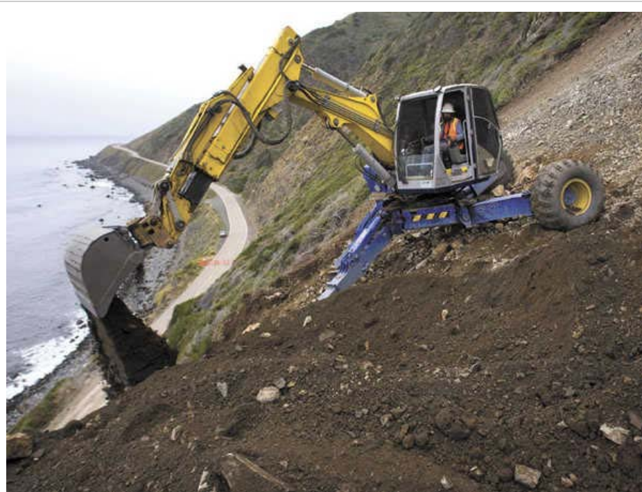
By David Middlecamp | dmiddlecamp@thetribunenews.com | purchase prints Some 200 feet above sea level on the steep slopes of the Alder Creek slide, Tracy Lemke shovels dirt using the Spider, a nimble piece of equipment designed for difficult terrain. In the background, Highway 1 heads north to Gorda. Click for more photos »
